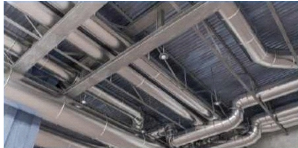
Can clean rectangular ducts
